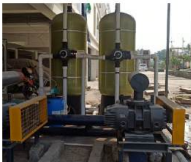
300 KLD for Samruddhi Apartments
