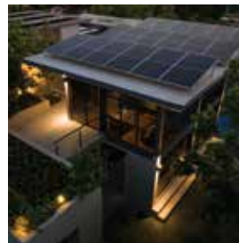
Solar Home Power
